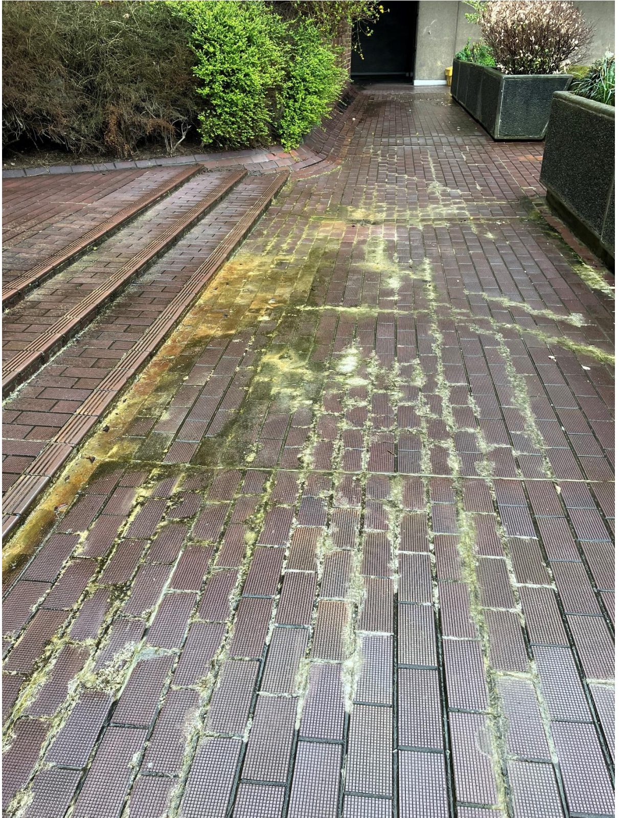
Image 4: Existing tiles have become degraded due to the water pooling.
